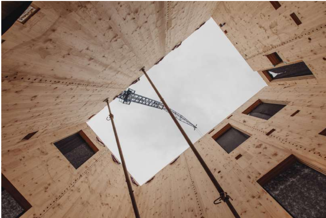
A tower of timber created using renewable materials and highly innovative construction methods. Photography courtesy of TOG.
